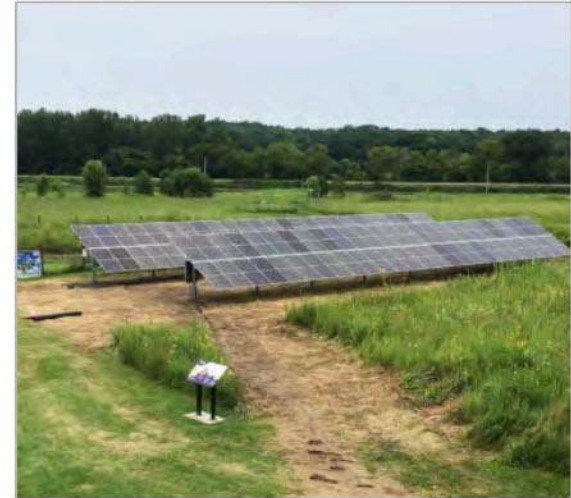
Solar array at Hurstville Interpretive Center. Photo Credit: Jackson County Energy District website
