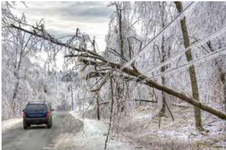
Ice storm impacts power lines
