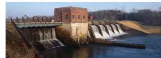
Maquoketa hydroelectric power plant. Photo Credit: http://renewableworldenergies.com
