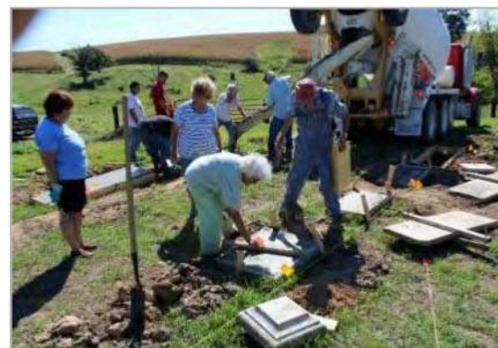
Commissioners and volunteers at work with the repair and restoration of a pioneer cemetery. Photo credit: Jackson County Pioneer Cemetery Commission Facebook page
